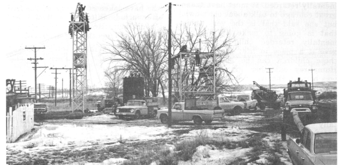
A GREAT DEAL OF ACTIVITY takes place as the Montana Power Company's crew is working on a 69,000-volt tiein line to the Wagner substation, the Bureau of Reclamation's crew installs metering equipment and the Big Flat Electric crew works on the erection of the new substation.
